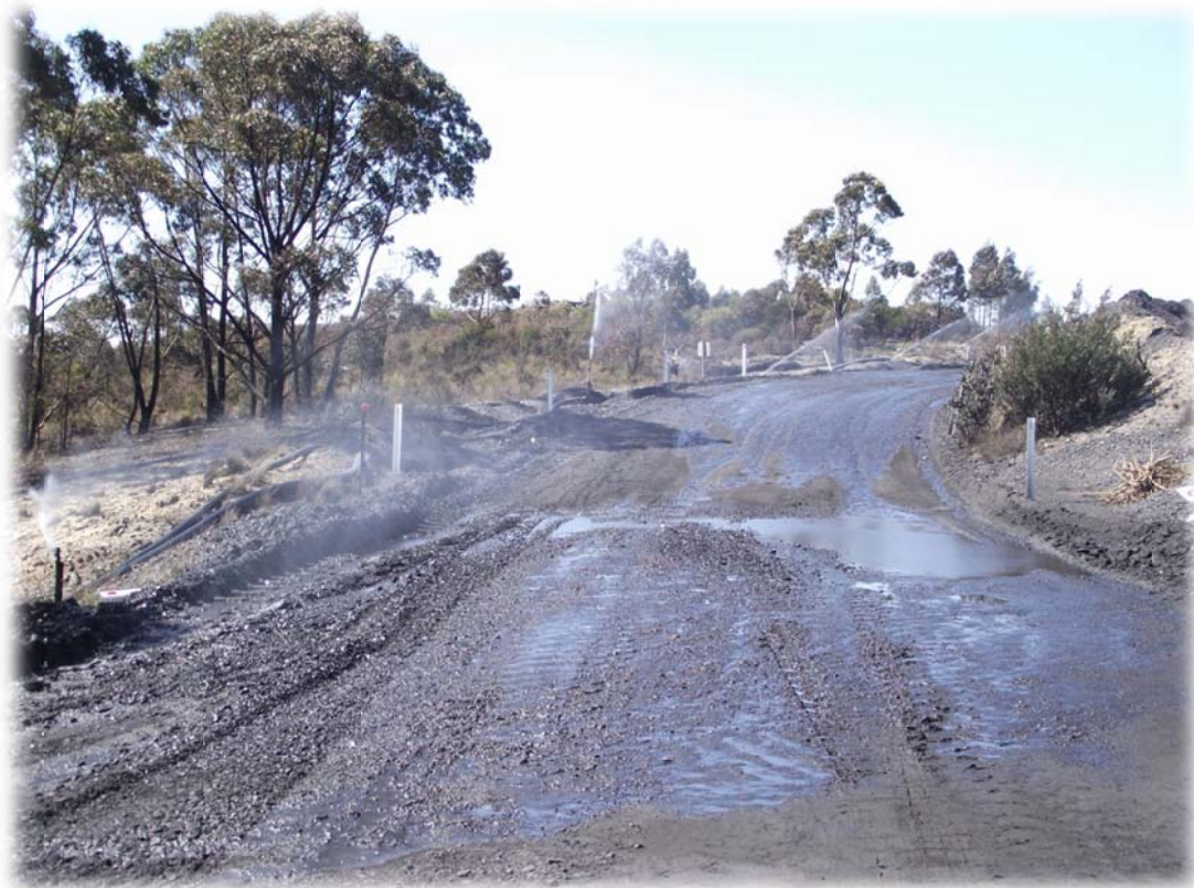
Figure 10 REA Haul Road Sprinklers
