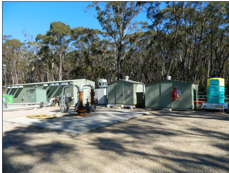
Plate 1 – Bore 6 Dewatering Facility
